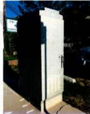
Traffic Signal Winter Canyon Road (b)
