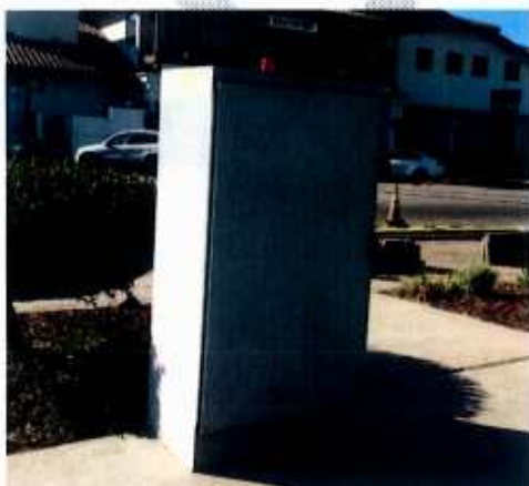
Waste Water Treatment Box (c)
