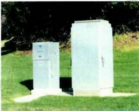
Traffic Signal Malibu Canyon Road (a)
